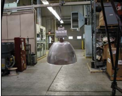
Old Style Lighting Fixture- 368 Watts
